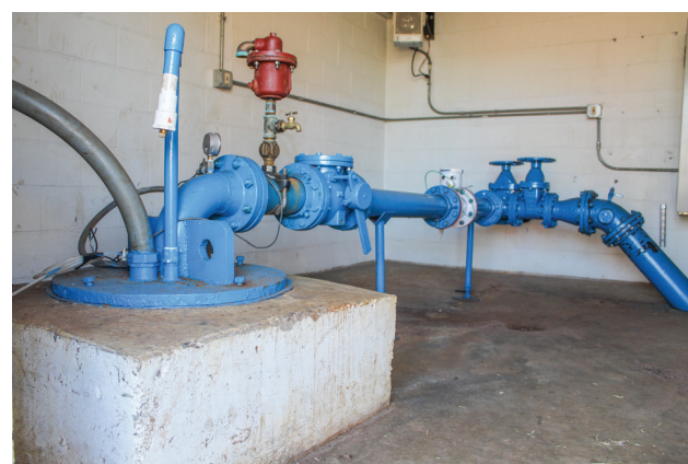
Mustang well 12 is located at SW 119th Street and Pennsylvania Avenue. Wells 12 and 2 will receive the new water filtering system in 2021. Photo / Haley Humphrey
